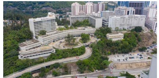
Source: Demolition of all existing buildings of Kwai Chung Hospital by Hospital Authority (2020)
